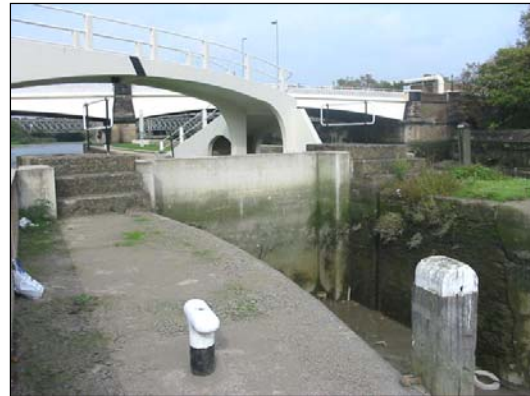
The sluice beside Bow Locks has not been in use for many years, but now the gate has been replaced by a solid slab of concrete and the channel is rapidly silting up.
