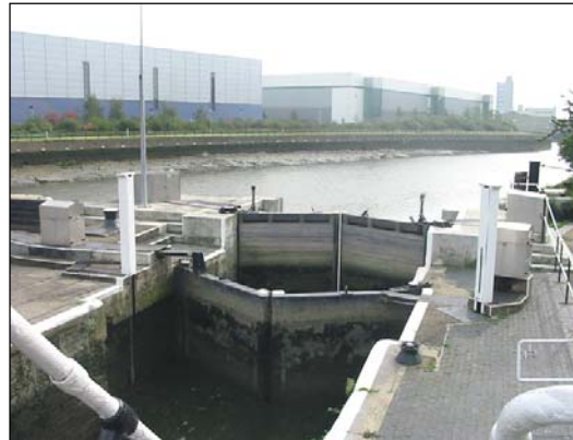
Additional outer gates have recently been added, and these can be left in the open position to allow 'free flow' through the lock.
